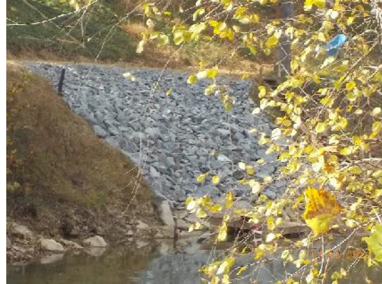
Figure 2: New rip rap installed just upstream from Darden Towe boat ramp at River right on a private property
